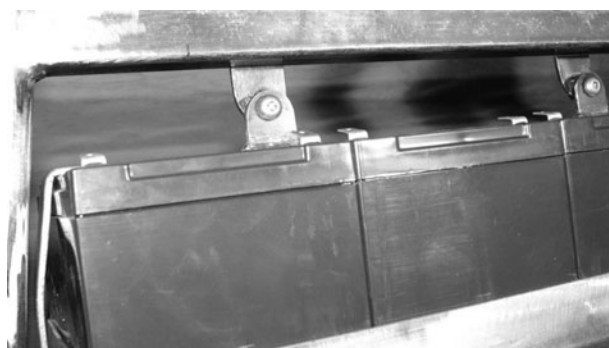
Figure 13-54 Battery pack securely mounted
